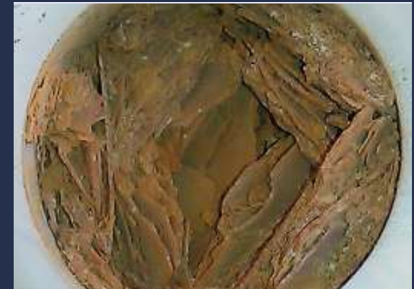
Clogged water plastic PPR (after cleaning the plate heat exchangers with chemicals).
